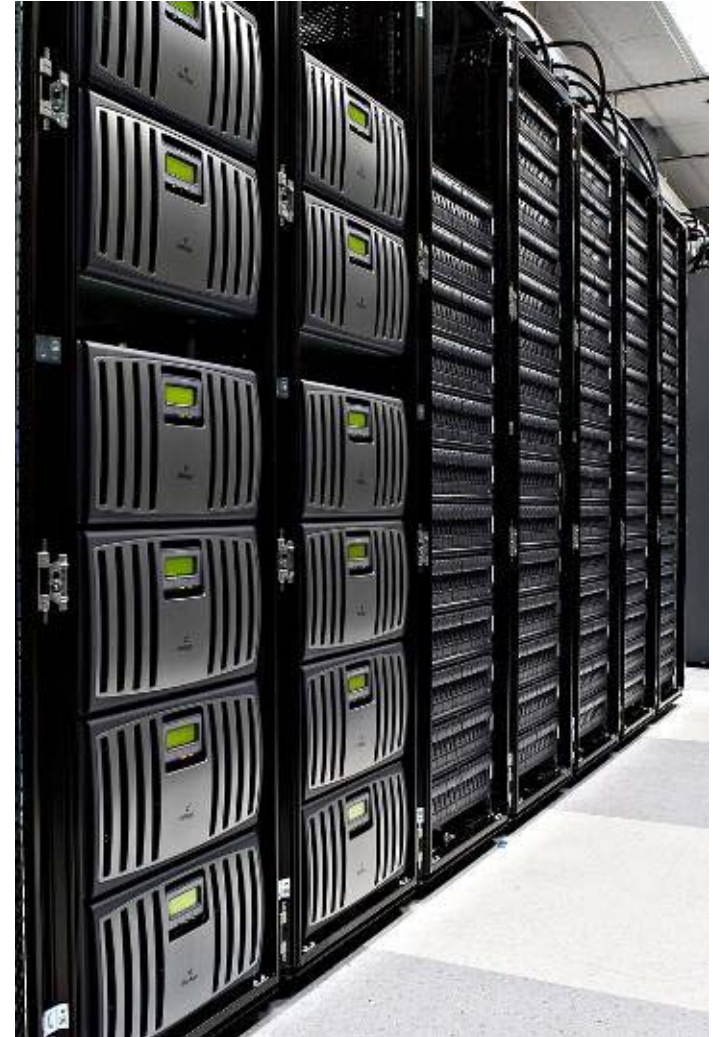
Engineering Data Center Lab
