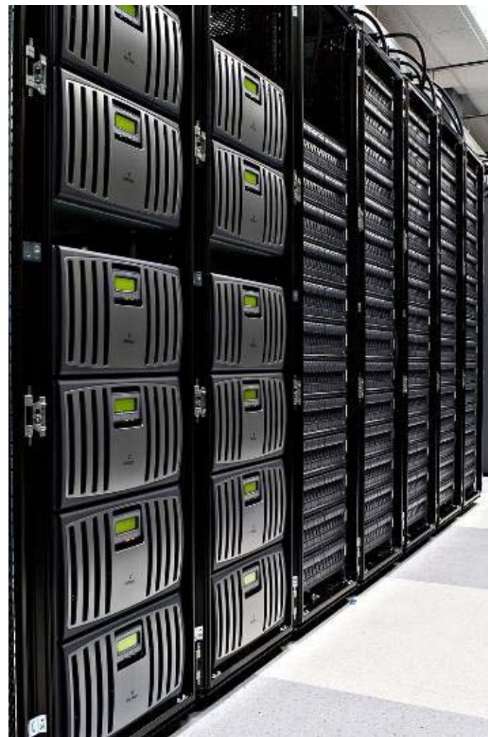
Engineering Data Center Lab
