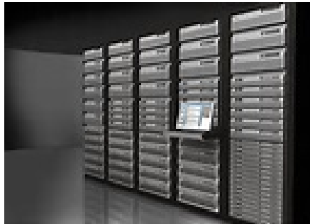
Storage Centers – Med Size (Centralized CSP and Telecom)
